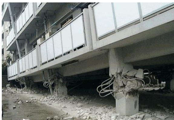
Fig. 1.1 Pilotis RC building damaged by shear-compression failure in Geiyo EQ (M=6.7), Hiroshima, 2001
