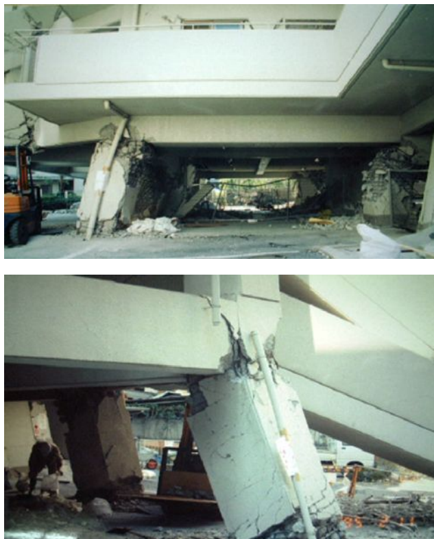
Fig1.2 Pilotis RC building damaged by flexural failure in Hyogoken-nanbu EQ (M=6.7), Hiroshima, 2001
