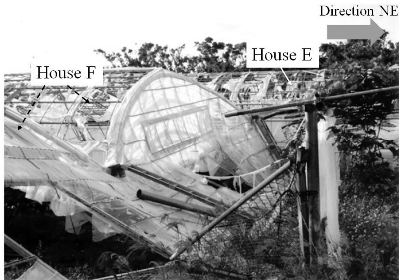
Fig. 3.9. Inclined gable end of house F (2 ream building).
