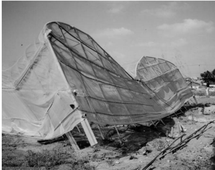
Fig. 3.14. Mode of collapse of greenhouse covered with net.
