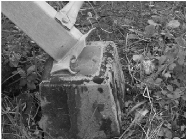
Fig. 3.8. Mode of collapse of base plate in pillar.
