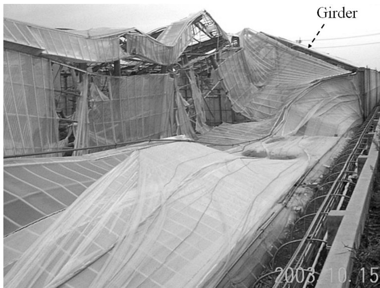
Fig. 3.3. Broken girder causing collapse of the roof of H beam steel plastic house.
