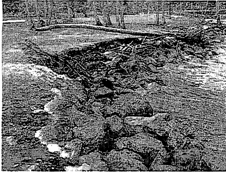
Erosion of Talafofo Bay
