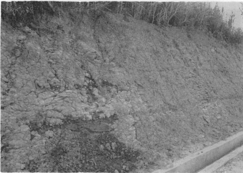
Picture—6 Seepage Outlet
