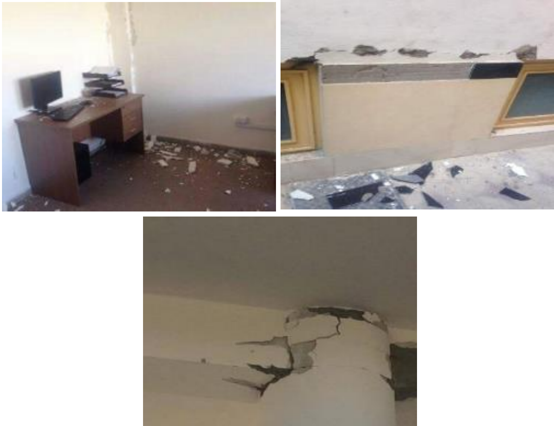
Figure 6.15 2015 Mw 7.5 Hindu Kush earthquake damage to reinforced concrete and masonry structures in Afghanistan
