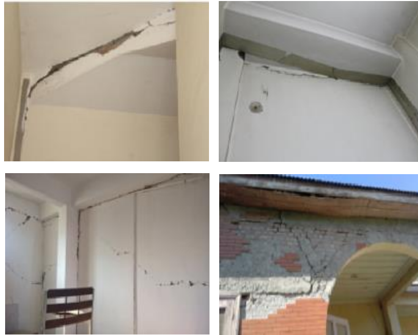
Figure 6.13 2015 Mw 7.5 Hindu Kush earthquake damage to reinforced concrete and masonry structures in Pakistan (Ahmed, 2015)
