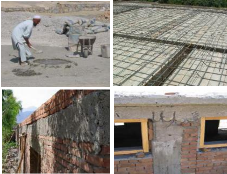
Figure 6.3 Concrete ingredients and hand mixing take place on a ground where the water and cement paste can penetrate. The reinforcement bending is in most of the cases poor. The bars are not wire-tied or welded on every joint. The wood panels and supports used for formwork is usually of poor quality resulting in wasting of cement water paste and insufficient space between the forms and reinforcement. The steel is exposed to atmosphere and the concrete is weak against water penetration.
