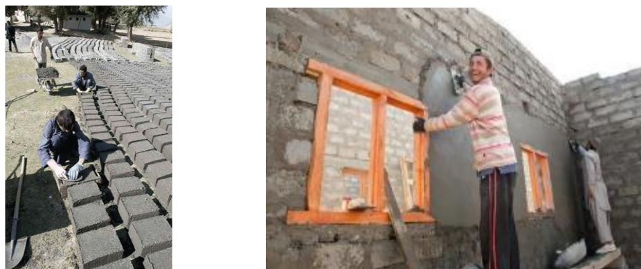
Figure 6.7 Producing and usage of CMU for a school building in northern parts of Afghanistan adjacent to the border with Tajikistan.
