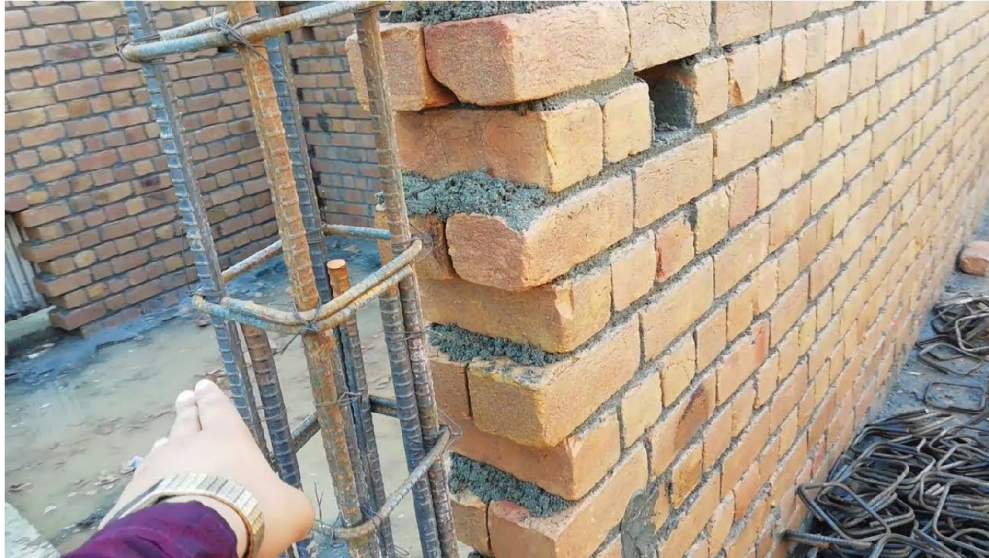
Figure 6.10 Formation of a rough surface to the end of the masonry so that it integrates well with the column.
