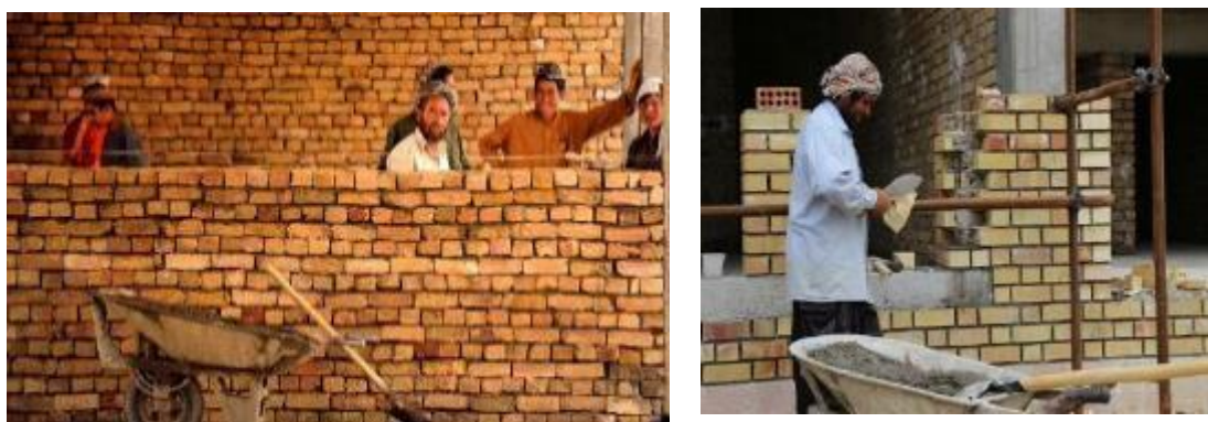
Figure 6.5 Brick masonry work with poor alignment of brick rows. A regular brick masonry work with high workmanship; however, this is not affordable by private owners and in government projects. (Gohar Khaton Girls School in Kabul).
