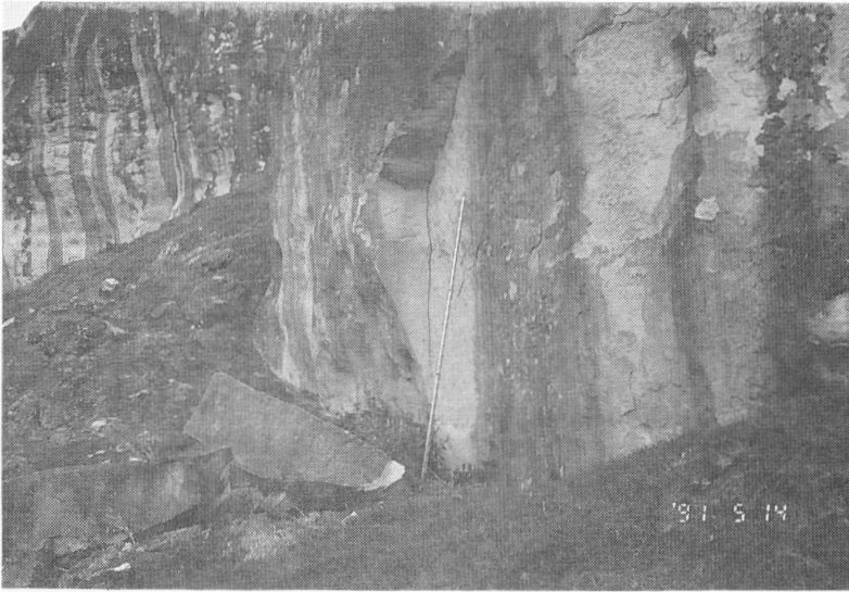
Photo 3. Glen Massey Sandstone bluff at Port Waikato Slope. Joints are parallel to the sandstone bluff. Sandstone blocks are found at the bluff foot.
