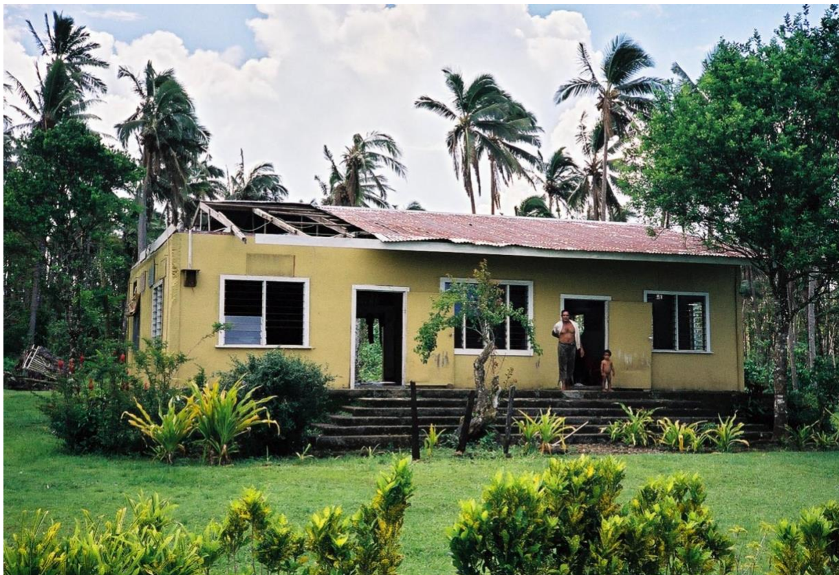
FIGURE 11. A Samoan family's damaged roof
